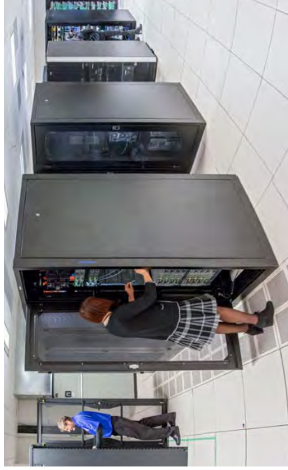
Figure 14: Regional server rooms. Cloud computing allows for data and applications to be centrally located and accessed by multiple devices
