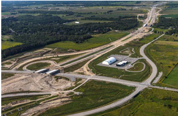
Figure 12: Highway 407, Phase 2 construction, looking southwest from the Bowmanville Avenue interchange (Source: Blackbird Infrastructure Group, August 2018)
