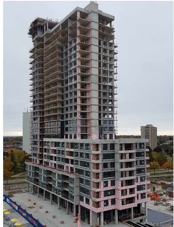
Figure 27: Market rental apartments under construction at Vision at Pat Bayly Square in Ajax, a project that received funding and support through Ajax’s Downtown CIP program, the Regional Revitalization Program and CMHC.
